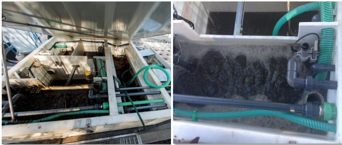
Figure 9. Presentation of the biological unit containing (from the left to the right) the MBR, aeration, anoxic and equalization tanks (left) and detailed view of the MBR tank (right).
