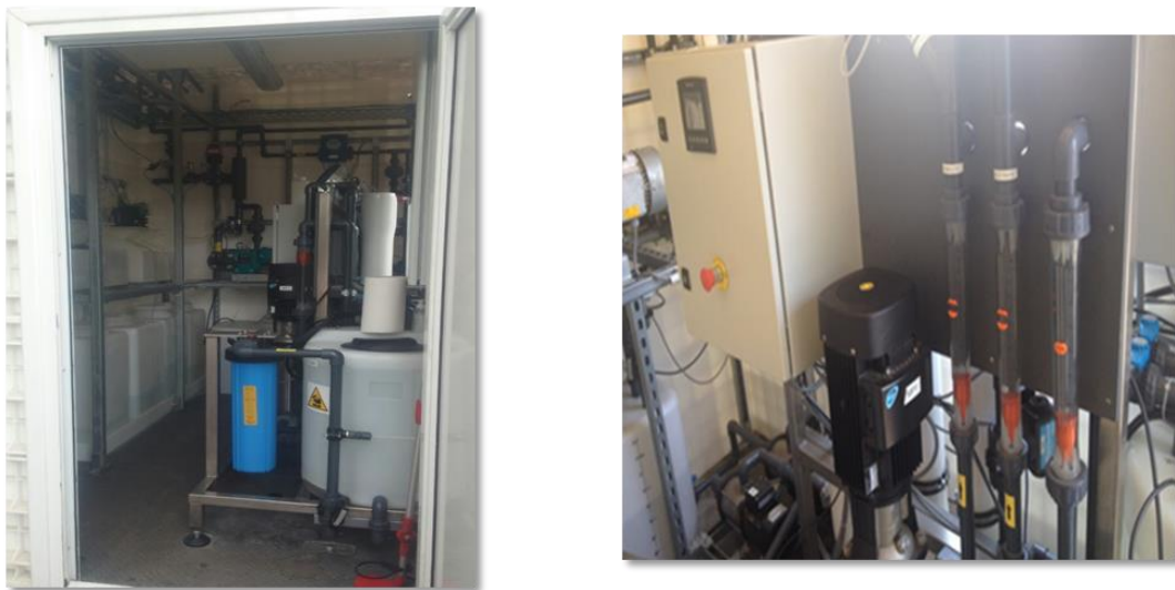
Figure 10. Presentation of the container that includes the RO unit and the electromechanical equipment (control room).
